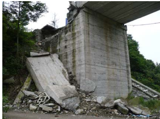
Fig 12. North abutment from the west. Note deck has moved west (or abutment moved east). IMG0476
