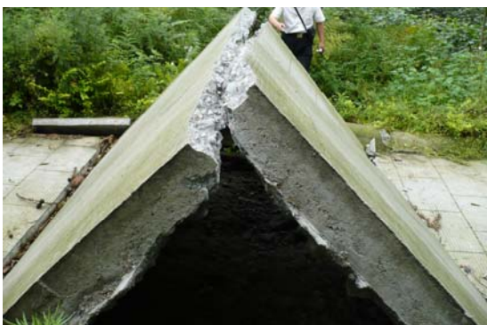
Fig 7. Buckling pathway pavement due to compression, of roughly 1m. Looking west. IMG0520
