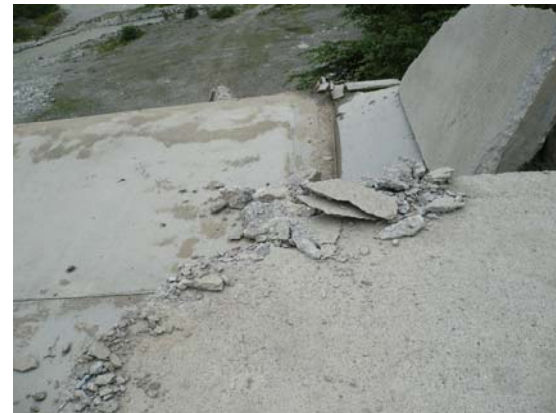
Fig 16. Displacement of north roadway over north deck, looking west. IMG0488
