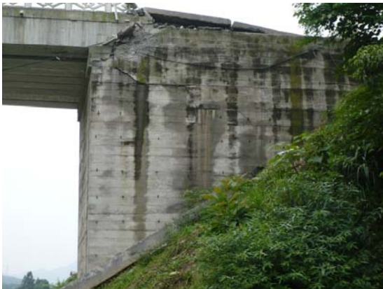
Fig 11. North abutment from the east. Note deck has moved north (or abutment moved south). IMG0463
