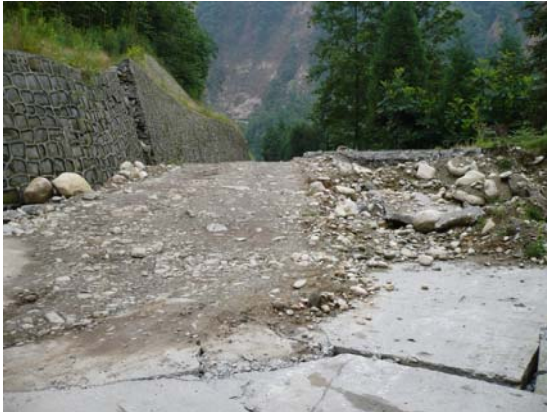
Fig 3. Extension of retaining wall along Chengxiang Road, Gao Yuan Village, looking roughly southeast. Note road has been filled in. IMG0502
