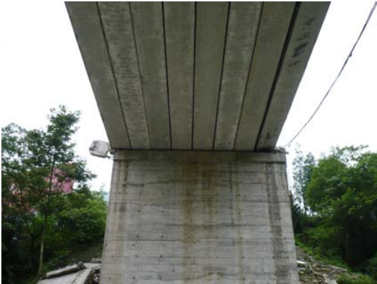
Fig 13. North deck, north end. Note displacement to the north and west. IMG0478
