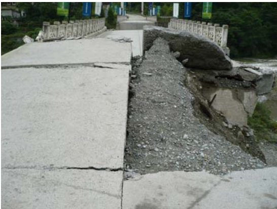
Fig 15. Heave and buckling of road on north abutment., looking south. IMG0483
