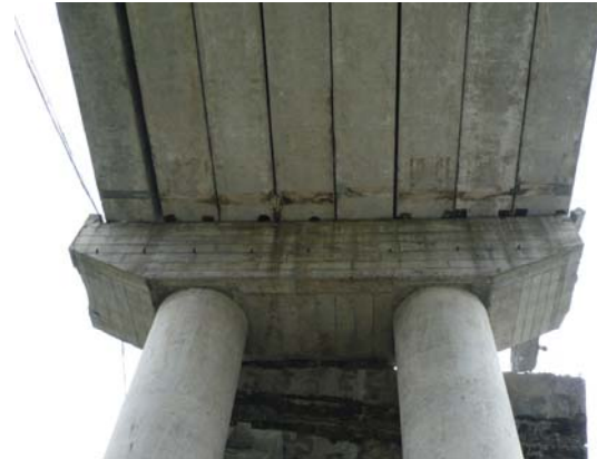
Fig 14. North deck, south end. Note deck has displaced to the north. IMG0479
