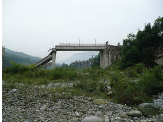
Fig 10. Gao Yuan bridge looking west, note displacement of north deck to the north. IMG0461
