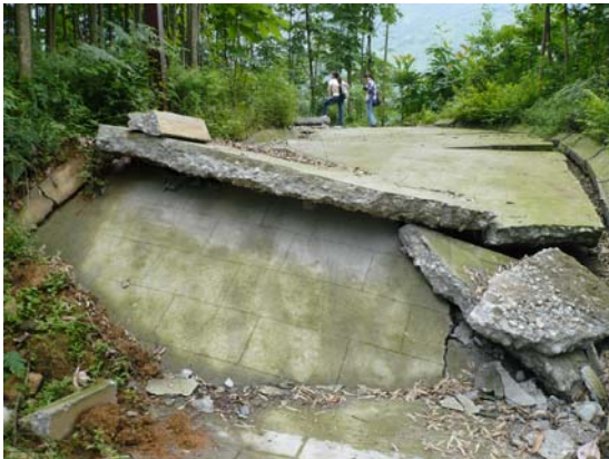
Fig 5. Permanent ground displacement along pathway. IMG0511
