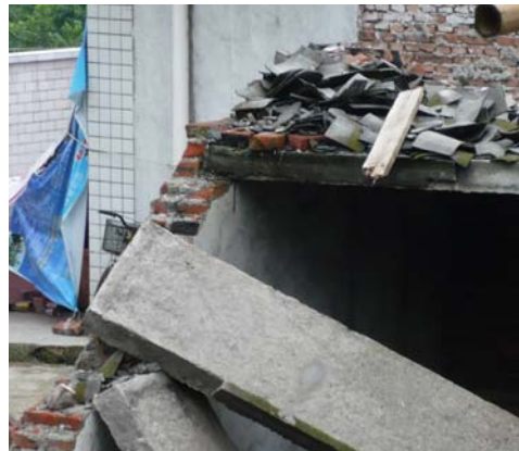
Fig 20. Lack of connection or confinement of precast concrete plank with URM wall, near Xiao Yu Dong Bridge. IMG0431
