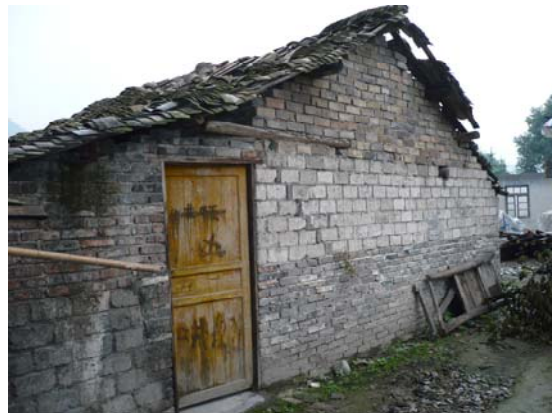
Fig 4. Unreinforced masonry house with brick and solid concrete block, displacement of clay tiles on roof, Danan Village. IMG0129
