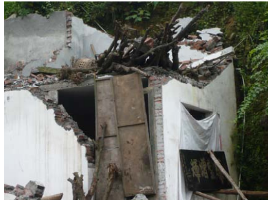
Fig 22. Partially collapsed two-story, rural unreinforced masonry with precast concrete plank floor and roof, near Xiao Yu Dong Bridge. IMG0436
