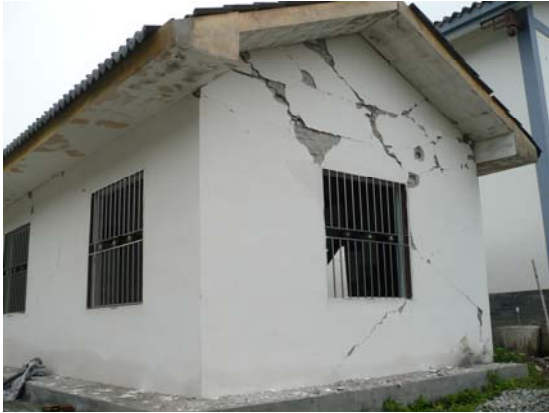
Fig 15. In-plane damage to unreinforced masonry building, Gao Yuan Village. IMG0569
