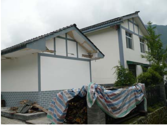
Fig 13. Single story URM with timber roof, cracked gable wall (two story building is confined masonry, described later) Gao Yuan village. IMG0559
