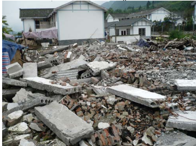
Fig. 2. Debris from collapse of unreinforced masonry buildings with precast concrete roof/floor planks (foreground), and 2-story confined masonry buildings with no damage (background) built in 2006 reportedly according to the Chinese Seismic Code. Gao Yuan Village, Wenchuan County
