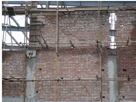
Fig 26. Confined masonry exterior wall for industrial building under construction, note tothing and steel connection between column and wall, near Pengzhou. IMG0347
