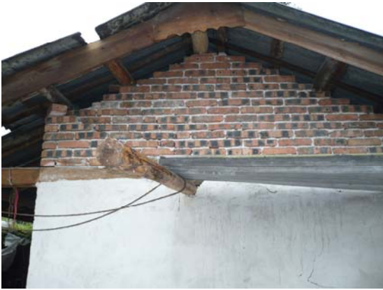
Fig 7. Crack in masonry gable wall, Danan Village. IMG0116
