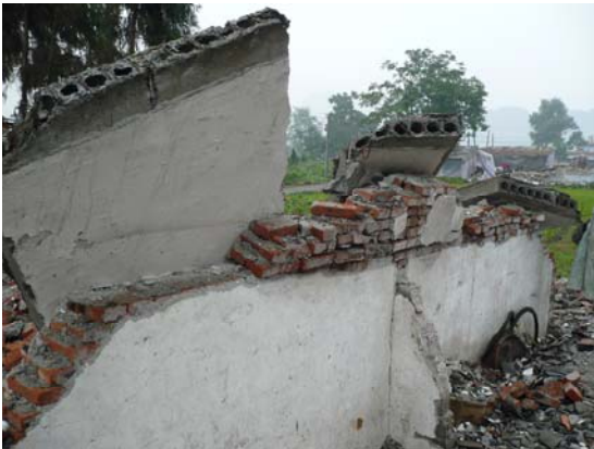
Fig 21. Collapsed two-story, rural unreinforced masonry with precast concrete plank floor and roof, Danan Village. IMG0085
