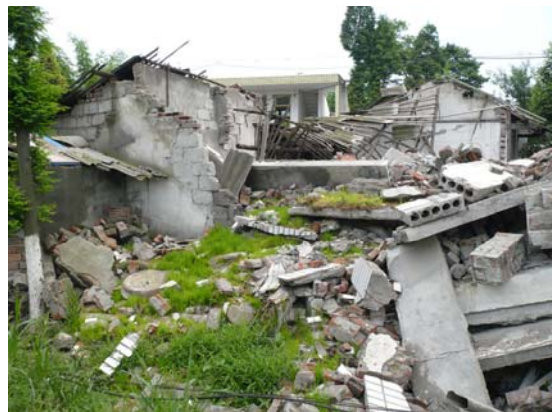
Fig 6. Partially collapsed unreinforced masonry with timber roofs in background, collapsed URM with concrete plank in foreground. Rural Pengzhou. IMG0351
