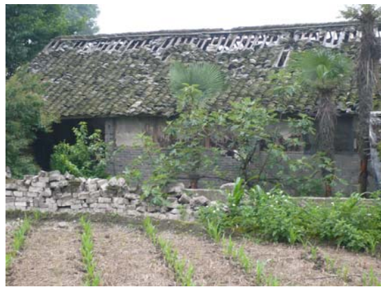
Fig 12. Typical traditional roofing system with simple clay tiles, free to slide during shaking. IMG0094
