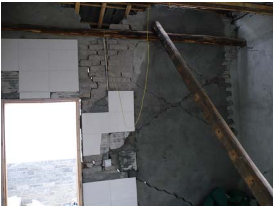
Fig 17. Damaged masonry wall not yet finished with ceramic tiles. Note cracks occur at the interface between brick and mortar. IMG0574
