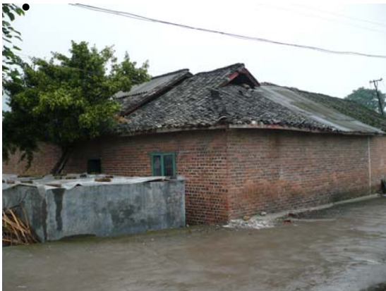
Fig 3. Unreinforced masonry house with pitched timber roof, no damage, Danan Village. IMG0104
